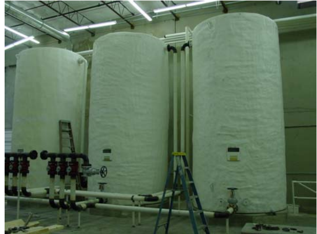
Three 6,000 gallon heated and insulated chemical tanks. Tanks, pumps, meters and piping installation by Smith Tank.
