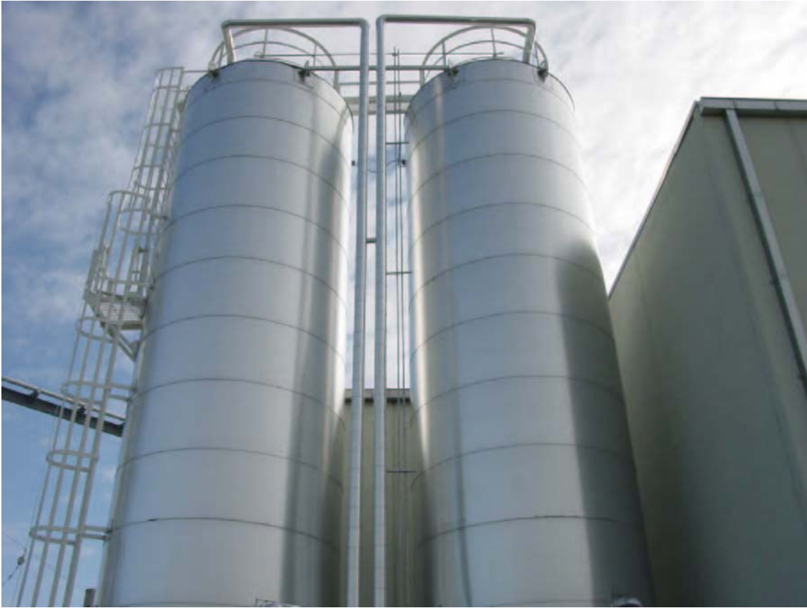
30,000 GALLON VERTICAL VEGETABLE OIL STORAGE TANKS
